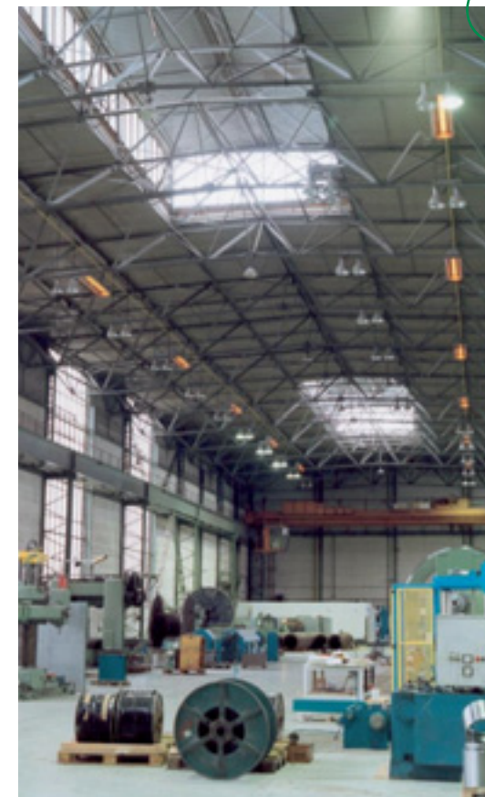
Heating of an industrial hall
